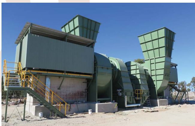
Ventilation Fans installed at Tritton Underground Mine over the new exhaust ventilation shaft
