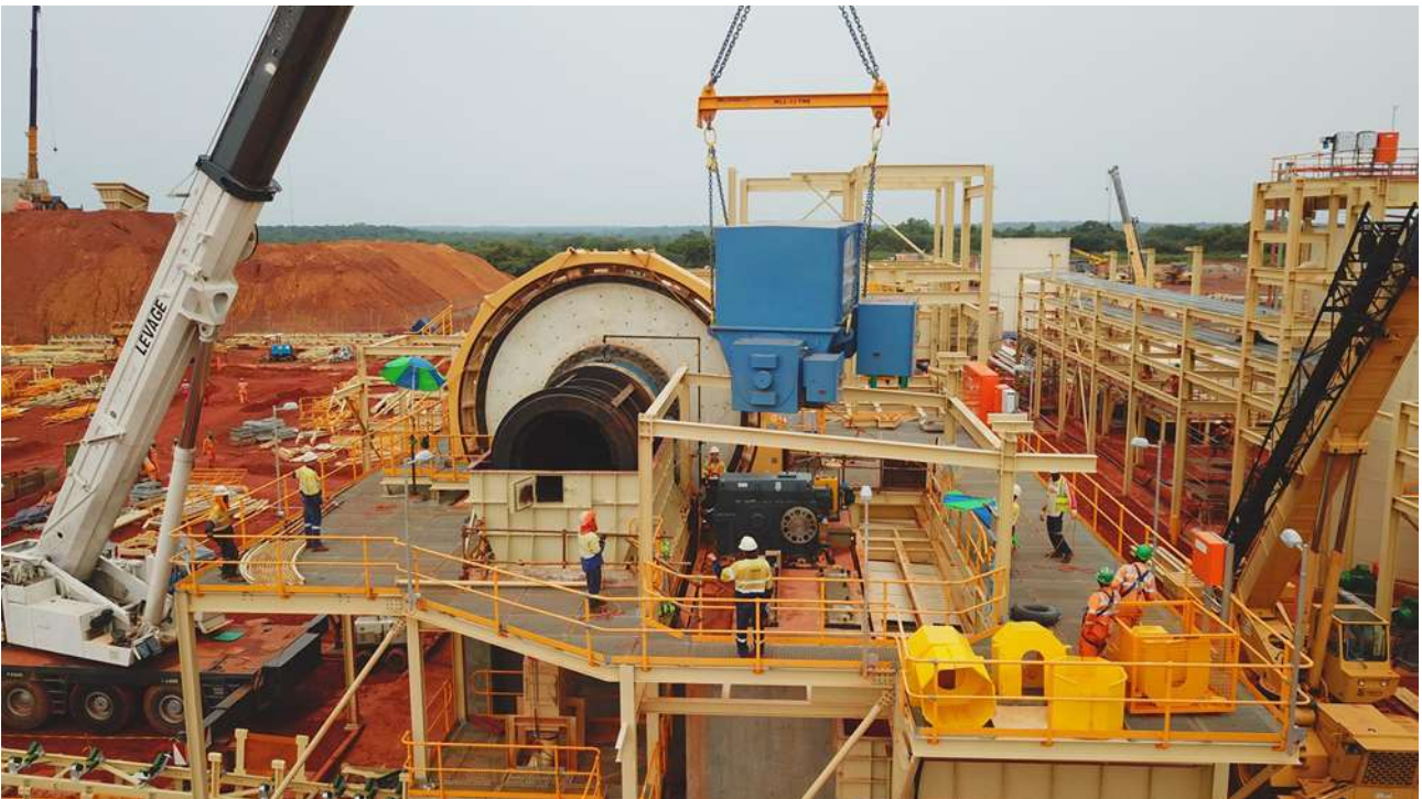
Erection of steel work and installation of plant for the grinding and CIL circuits is well advanced.
