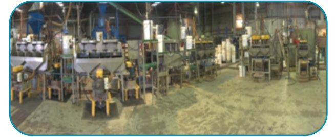
Flotation Pilot Plant Operation at ALS, Perth
