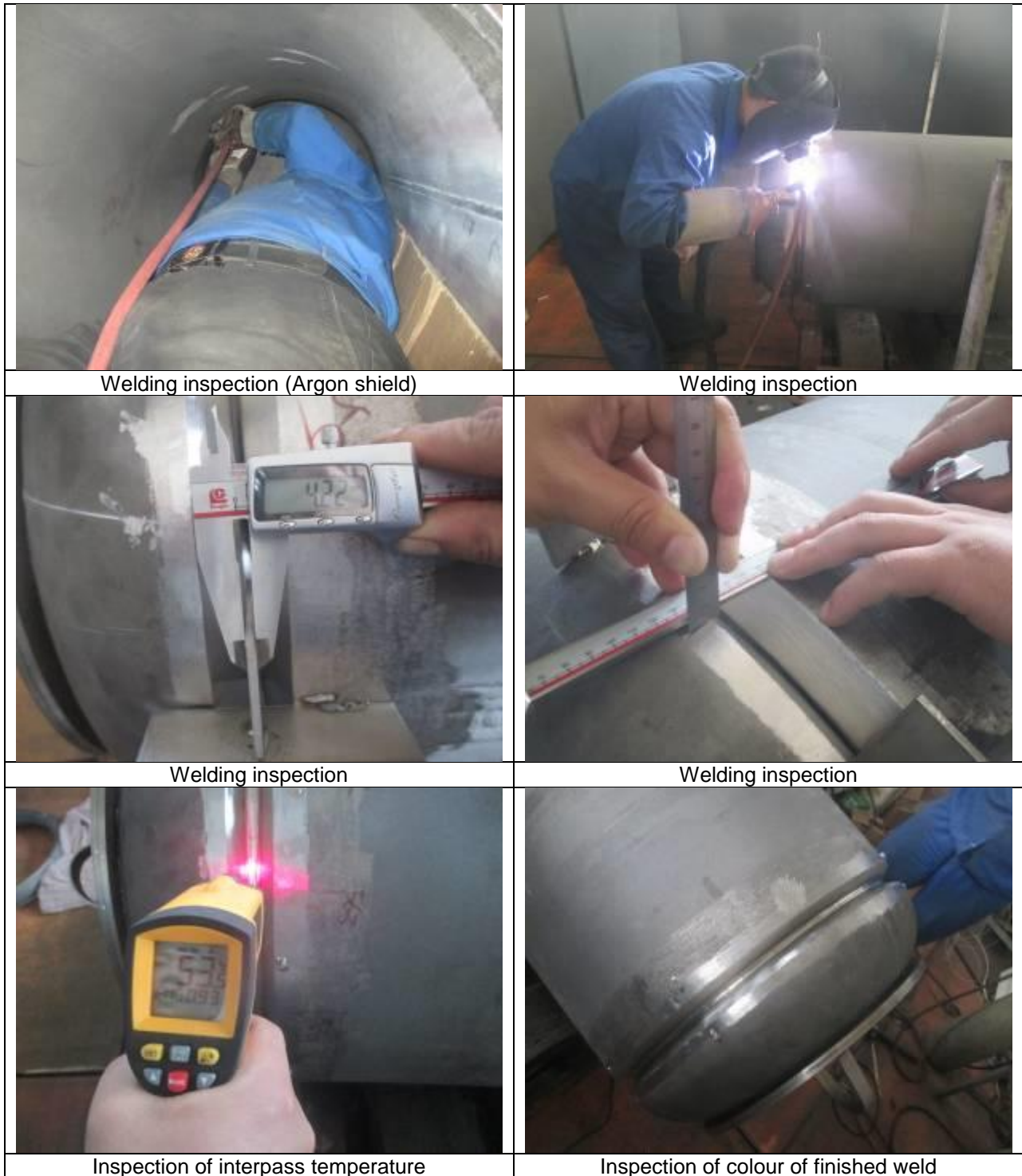
Figure 5: Inspection of the autoclave vessel bound for the demonstration-size processing plant in Perth, which has the capacity to process 2,200 kilograms of cobalt-nickel-scandium ore per day, producing up to 67 kilograms of cobalt sulphate, 500 kilograms of nickel sulphate and 8 kilograms of scandium oxide per week (when run on a continuous basis) 16 .
