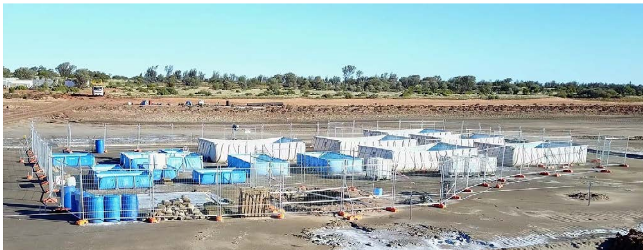
Figure 4: SET with both brine trains in operation
