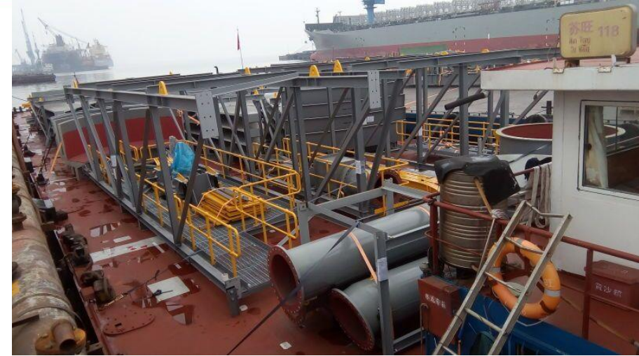
THICKENER MODULES – EX CHINA
