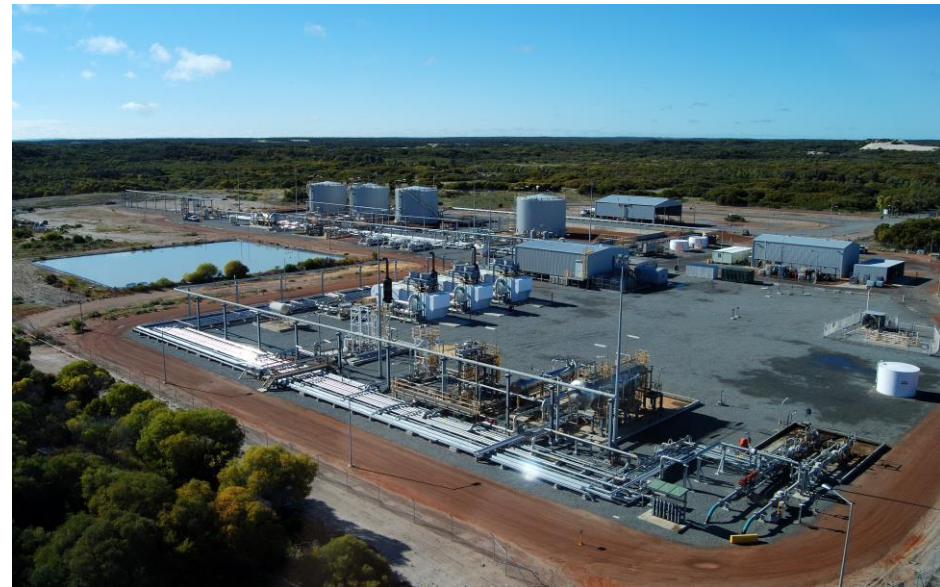
Arrowsmith Stabilisation Plant
