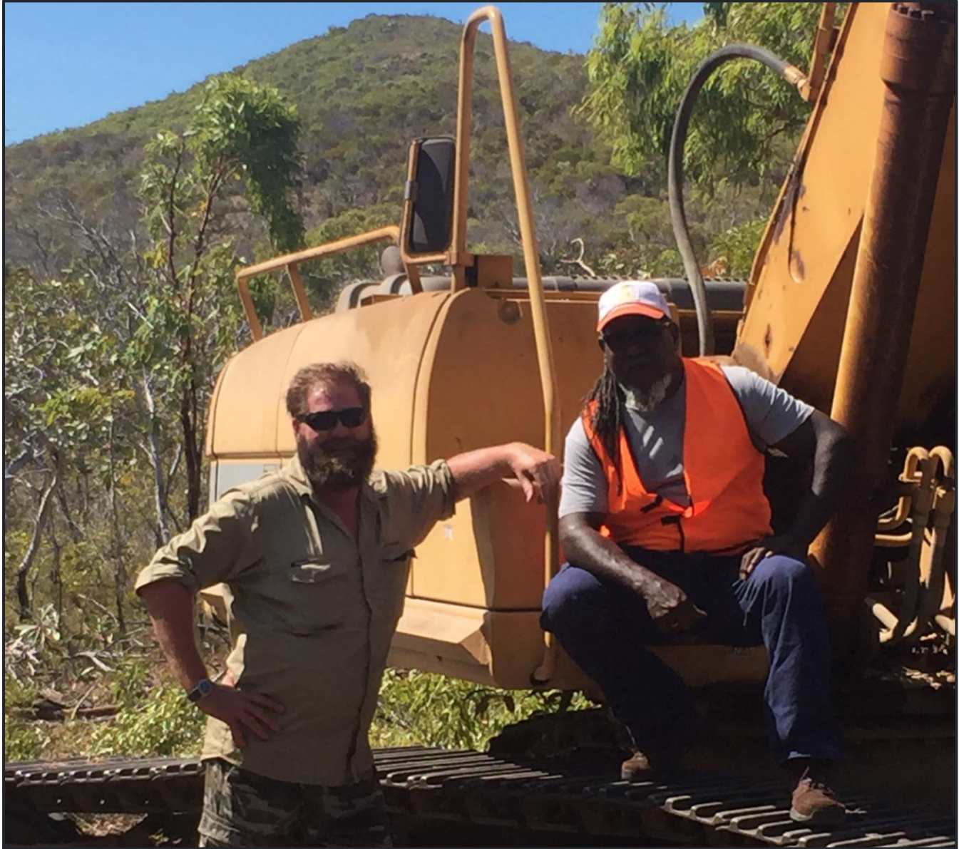
Figure 4. Sam Moody, company field technician and Milton Savage -Kaurareg Native Title Aboriginal Corporation during SSR site preparations.
