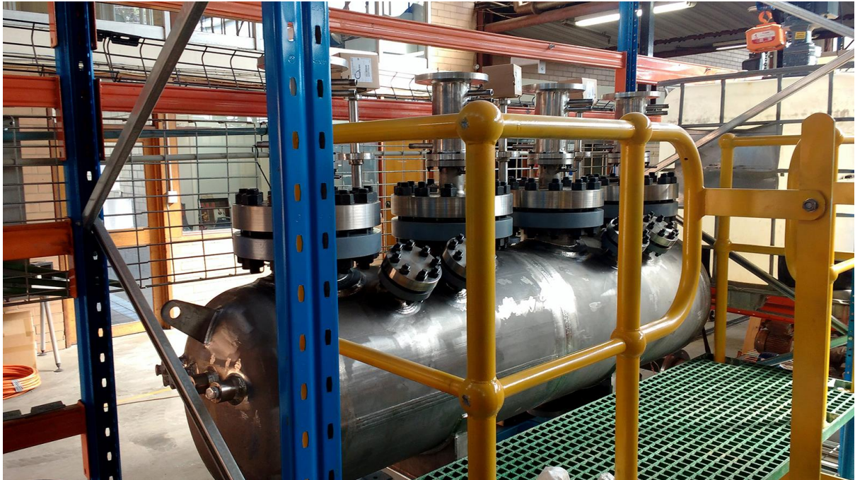
Figure 1: The autoclave has been installed as part of the demonstration-size plant, with commissioning scheduled to be completed in January. One of the world's leading inspection, verification, testing and certification companies completed a series of stringent quality assurance and control testing of the autoclave and subsequently certified that it complies with Australian standards.
