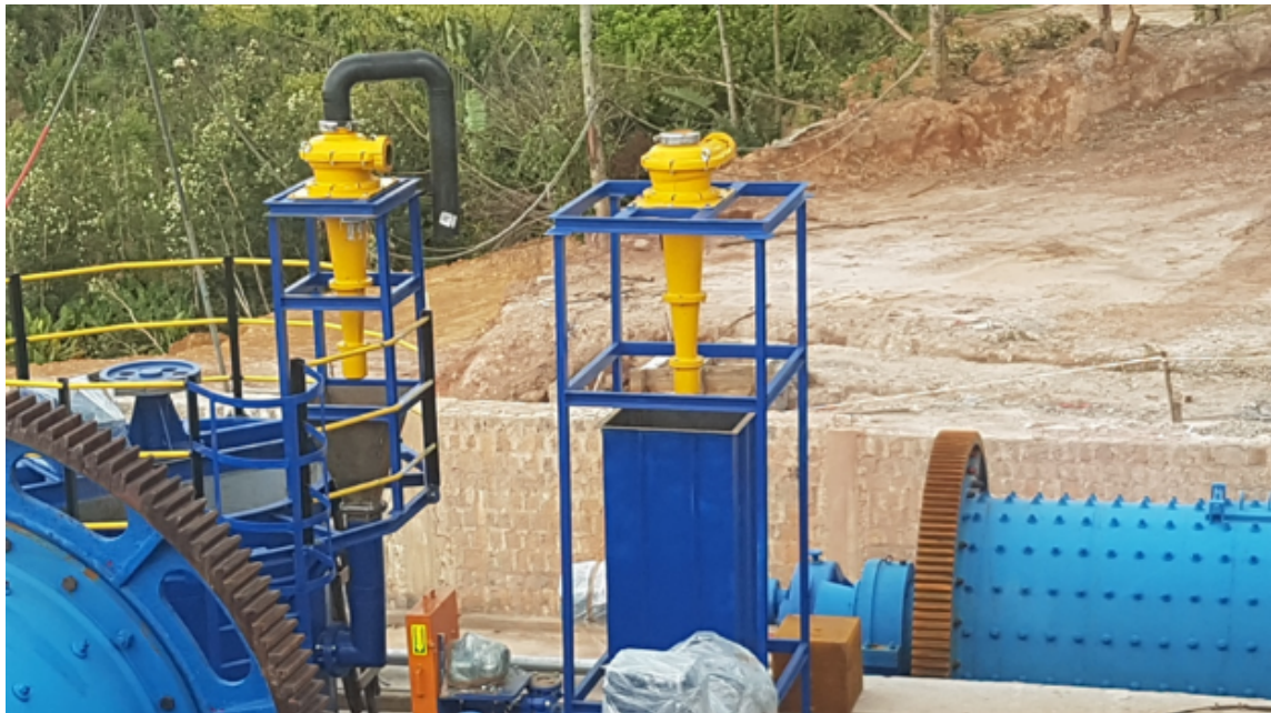
Process plant components ready for recommissioning.
