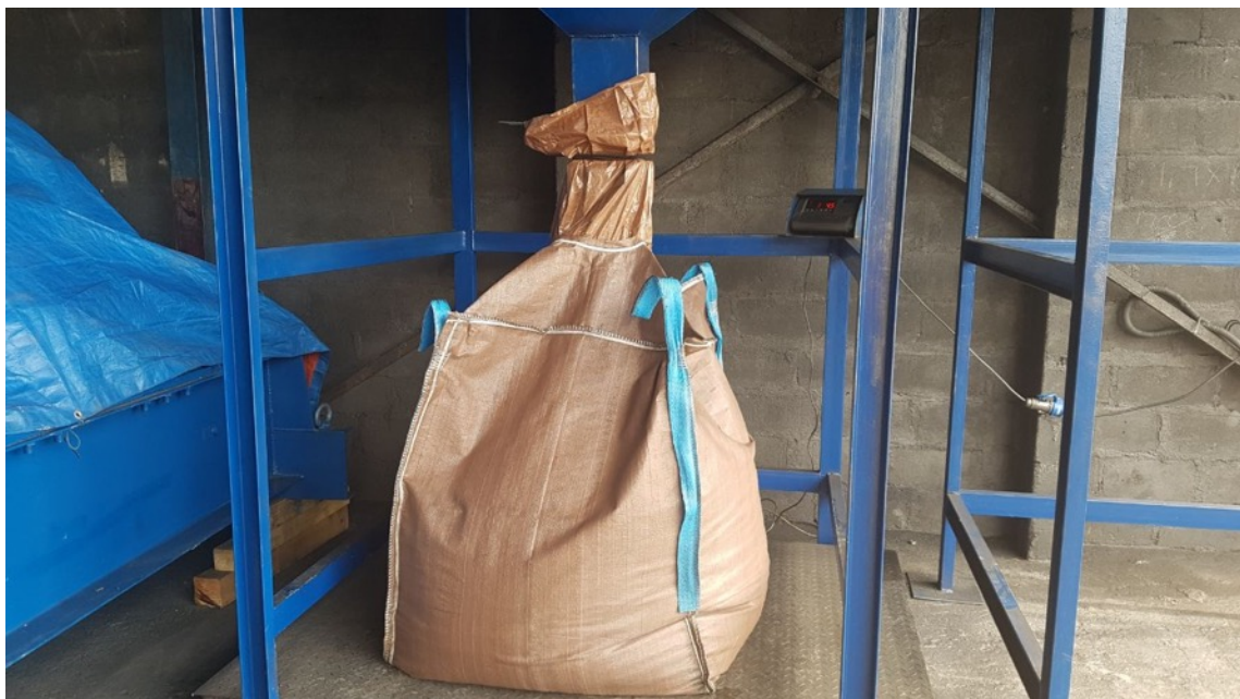
First concentrate from the recently commissioned Drying and Packaging system.
