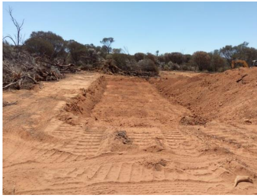
Figure 10. Excavation at Mertondale for some of the large nuggets including the 21oz nugget
