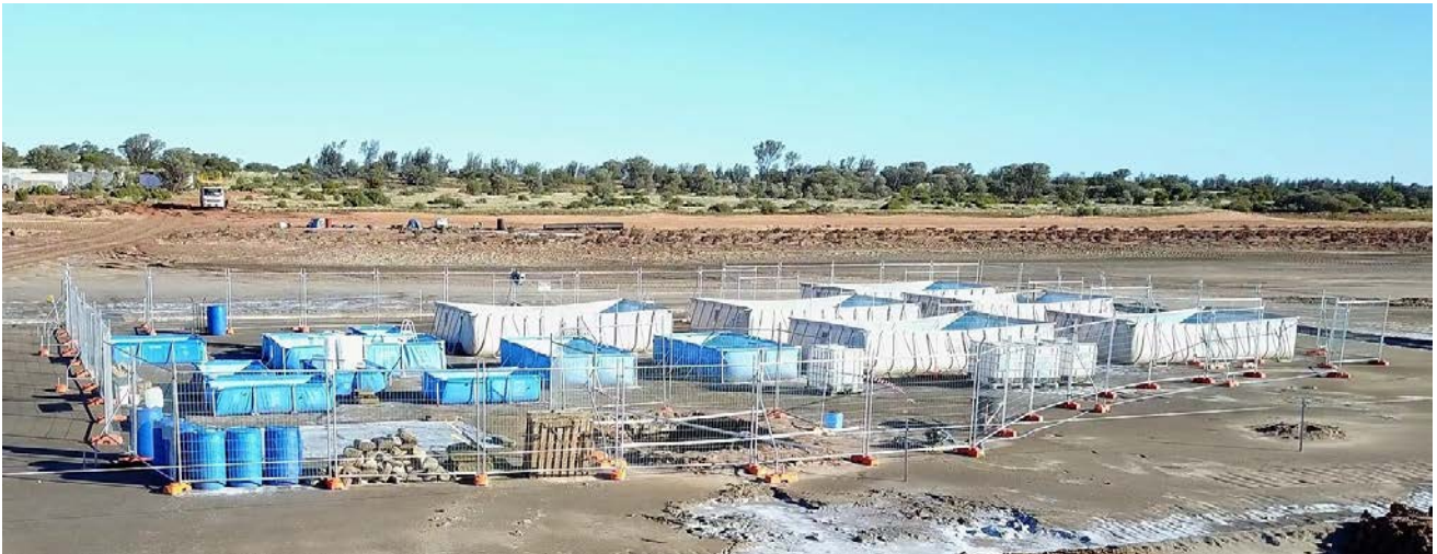
Figure 6: SET with Both Brine Trains in Operation
