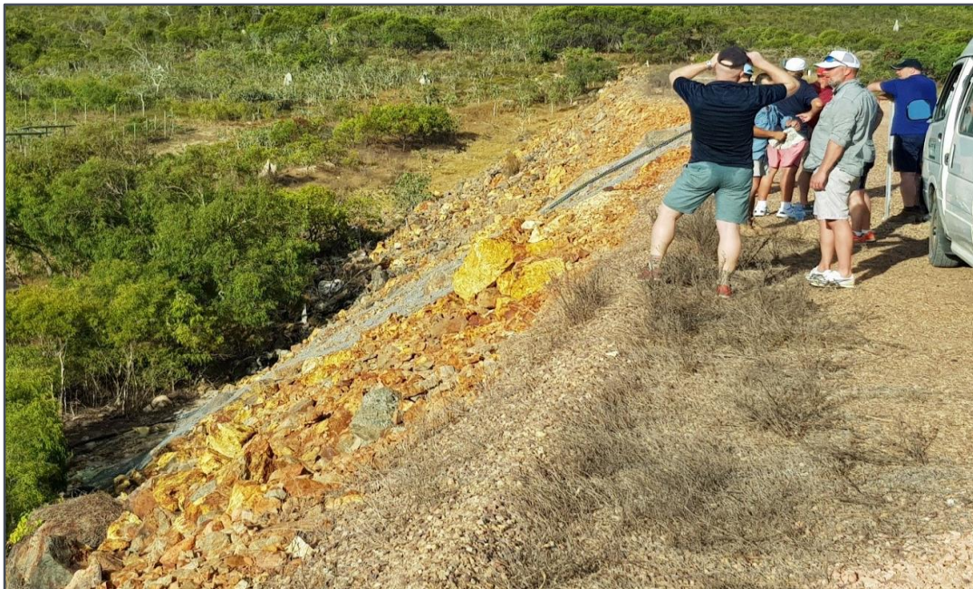
Figure 4. Loose rock construction of the process water dam wall. The yellow and brown stained rocks are related to oxidation of sulphides. High sulphides are often conducive to good gold values.
