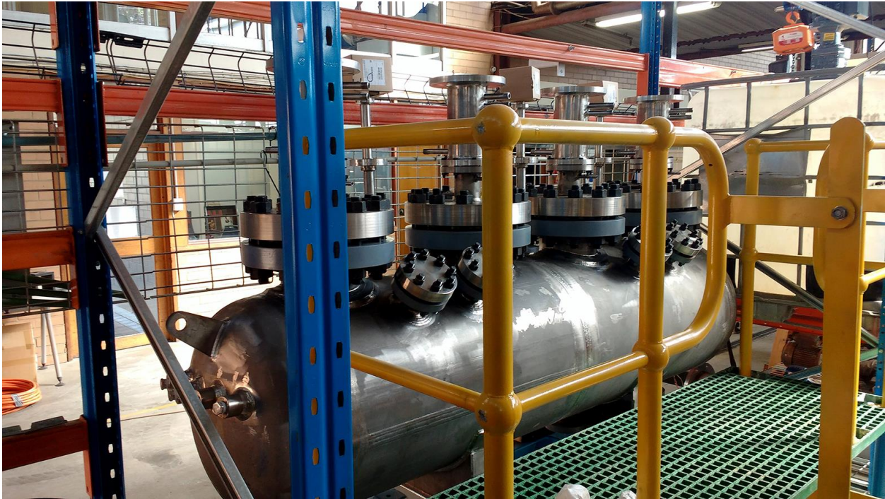
Figure 3: The autoclave vessel was delivered and installed at Simulus Laboratories Welshpool facility in Perth over the Christmas and New Year period. The autoclave has the capacity to process 2,200 kilograms of cobalt-nickel-scandium ore per day, producing up to 67 kilograms of cobalt sulphate, 500 kilograms of nickel sulphate and 8 kilograms of scandium oxide per week (when run on a continuous basis).
