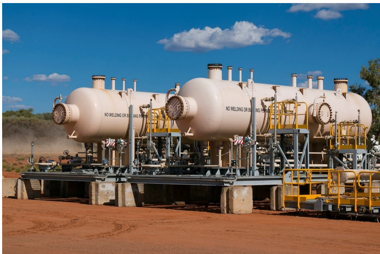
Figure 3: 2 out of the 3 separators purchased from Santos at Mereenie
