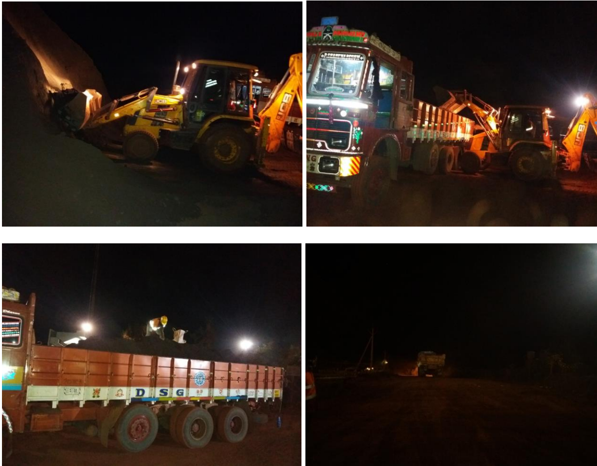
BMM Truck loading and dispatch
