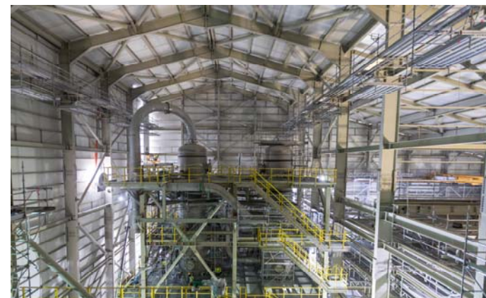
Pressure Oxidation Heat Recovery
