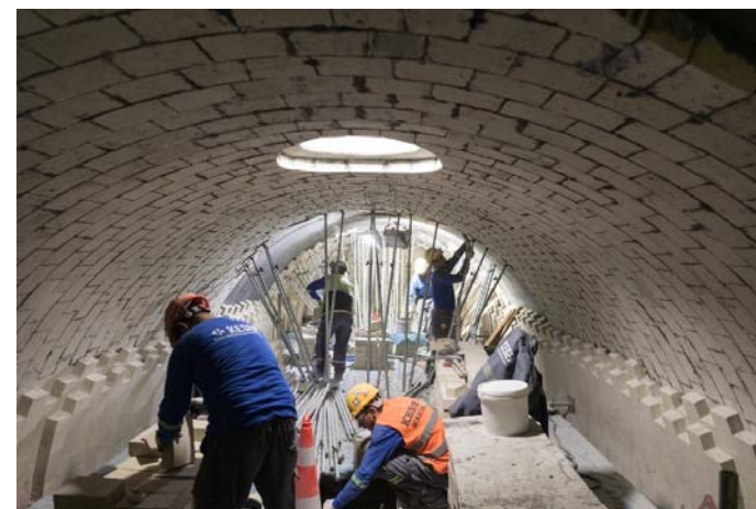
Autoclave Brick Lining
