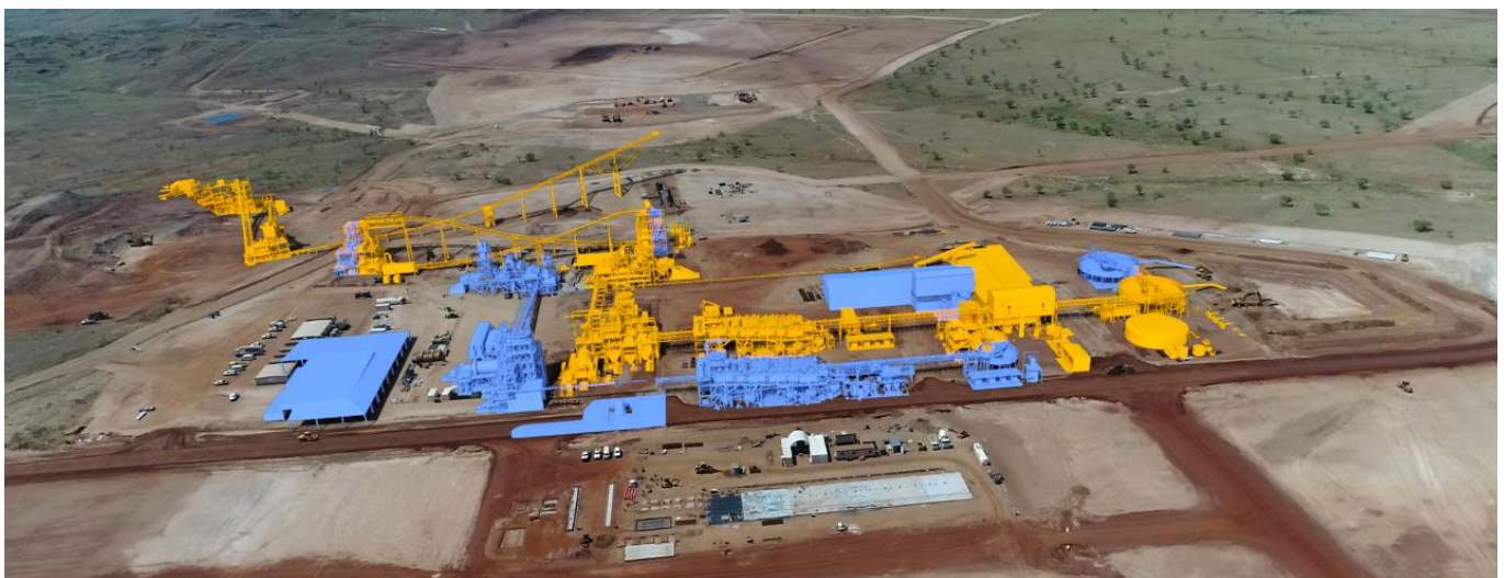
Figure 1 – Aerial photograph of current construction progress with Stage 2 3D model overlay (Stage 1 shown in orange, Stage 2 shown in blue)
