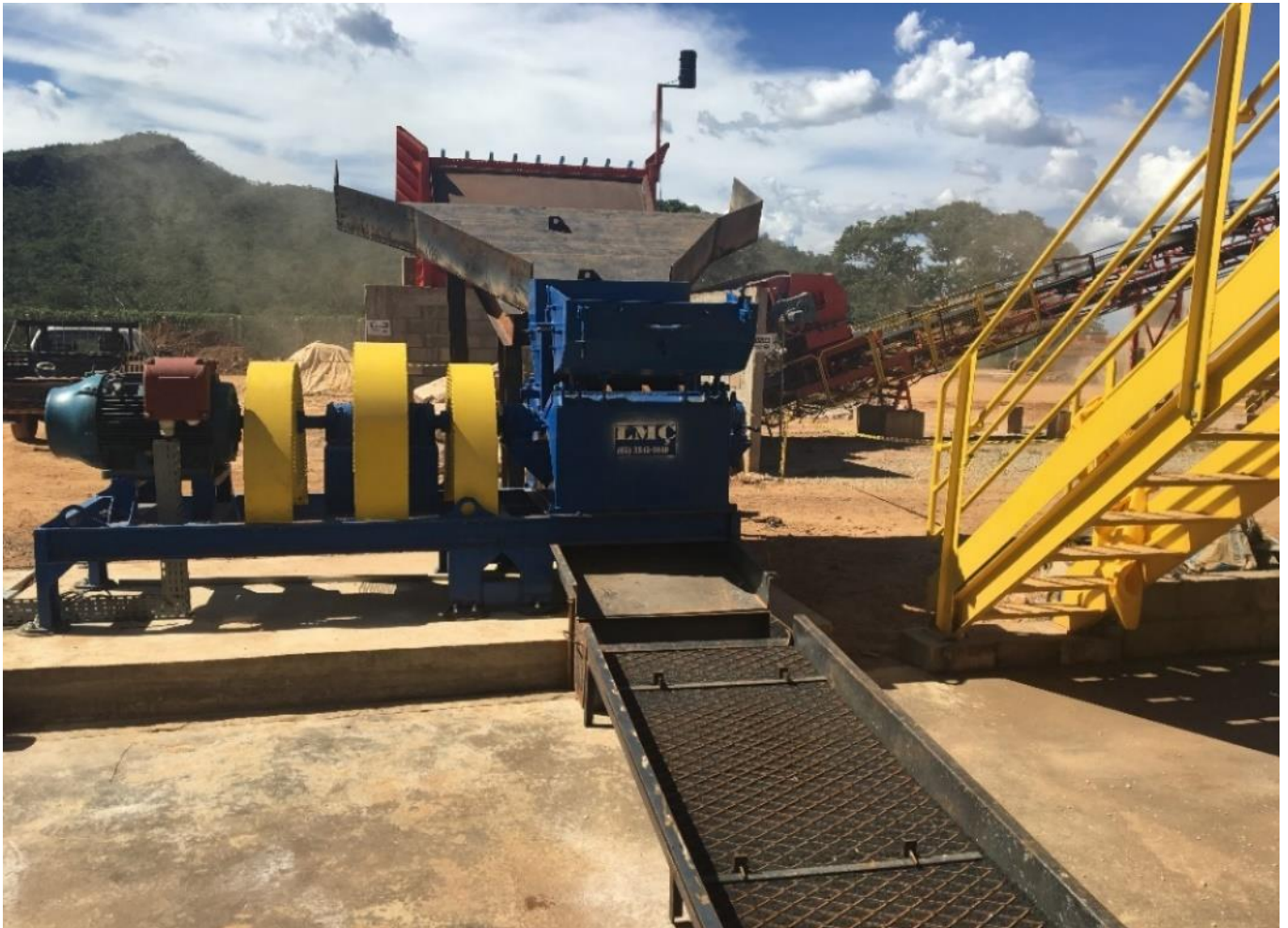
Image 3; Hammer mill installed
