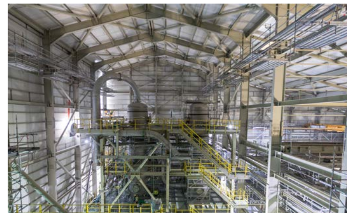
Pressure Oxidation Heat Recovery
