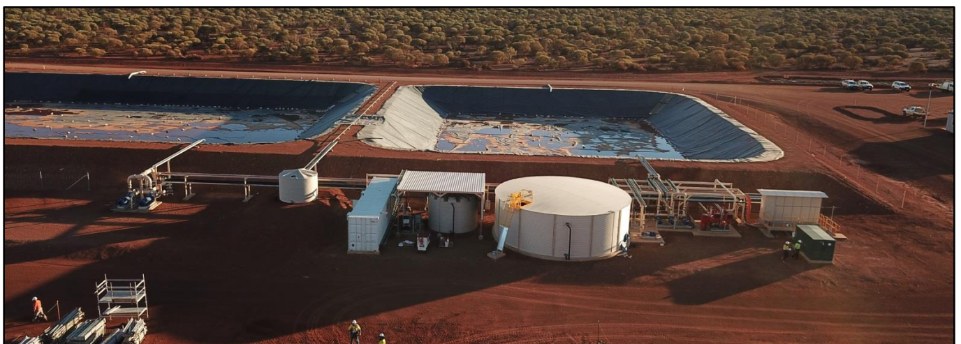
Photo 5: Water Services Area –Commissioned and Handed Over to Operations Team
