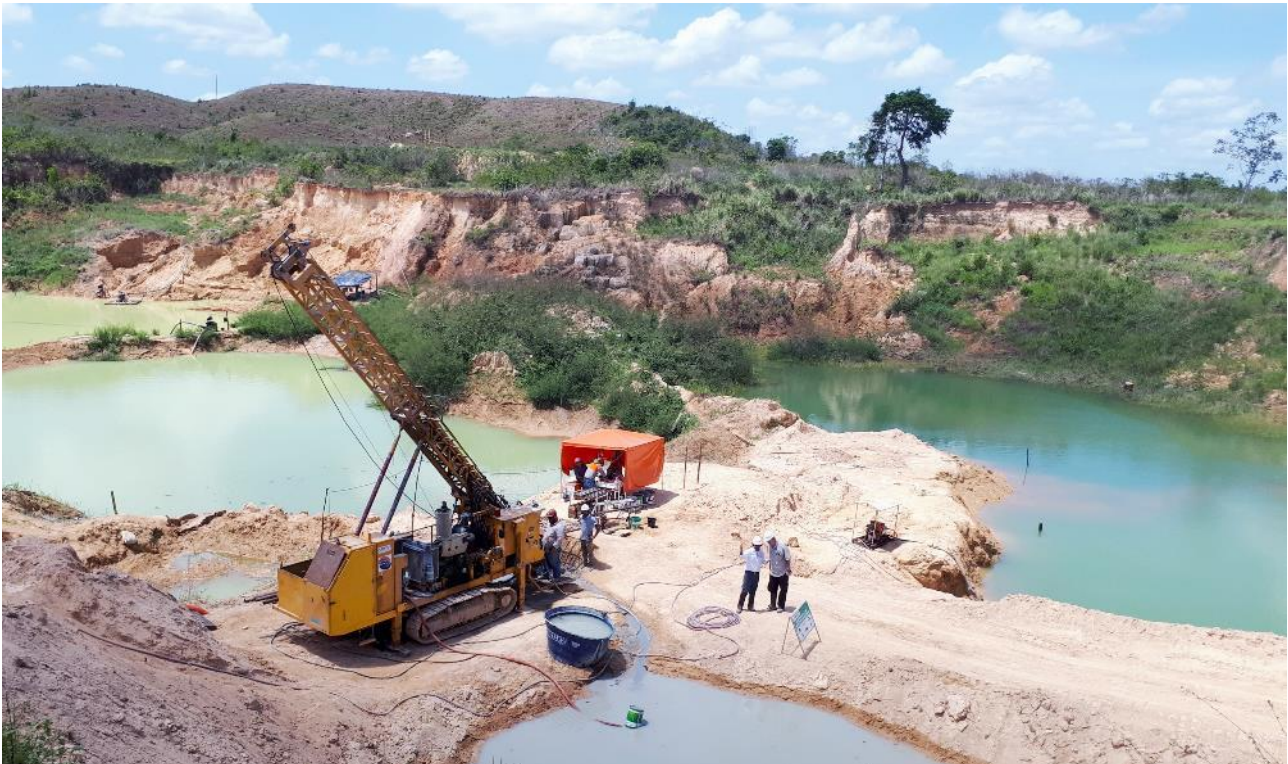
An example of drill access created inside historic artisanal workings at Contact
