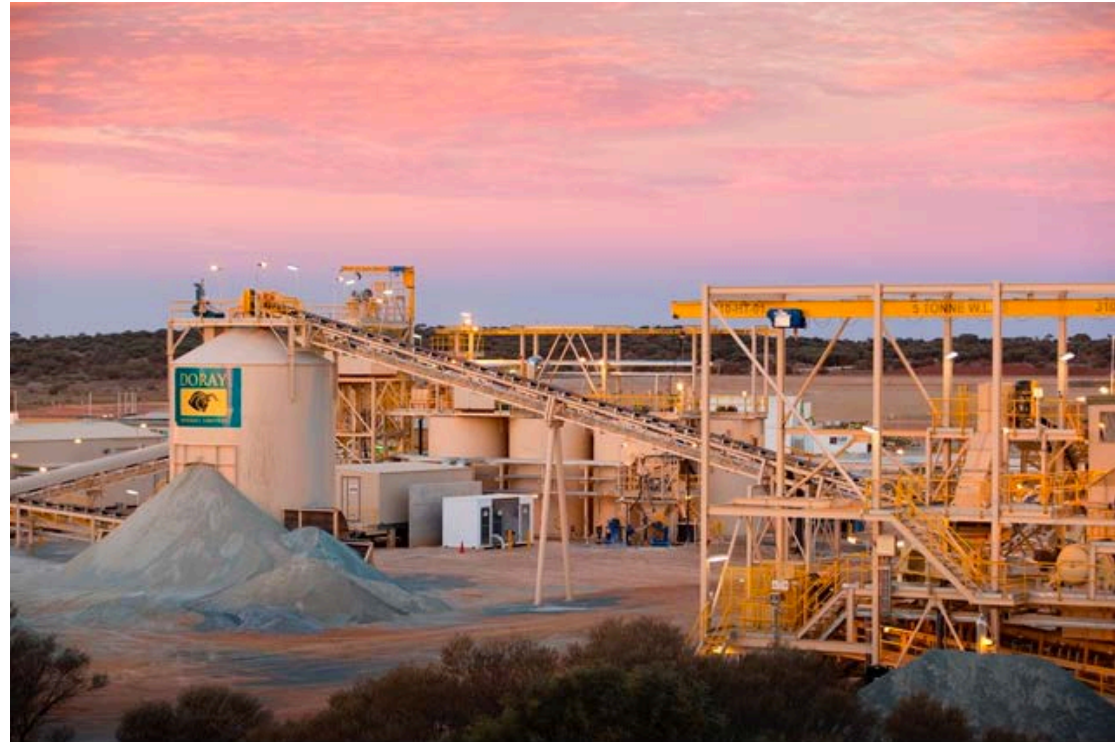
Doray Minerals Andy Well Gold Plant construction and design by GR Engineering
