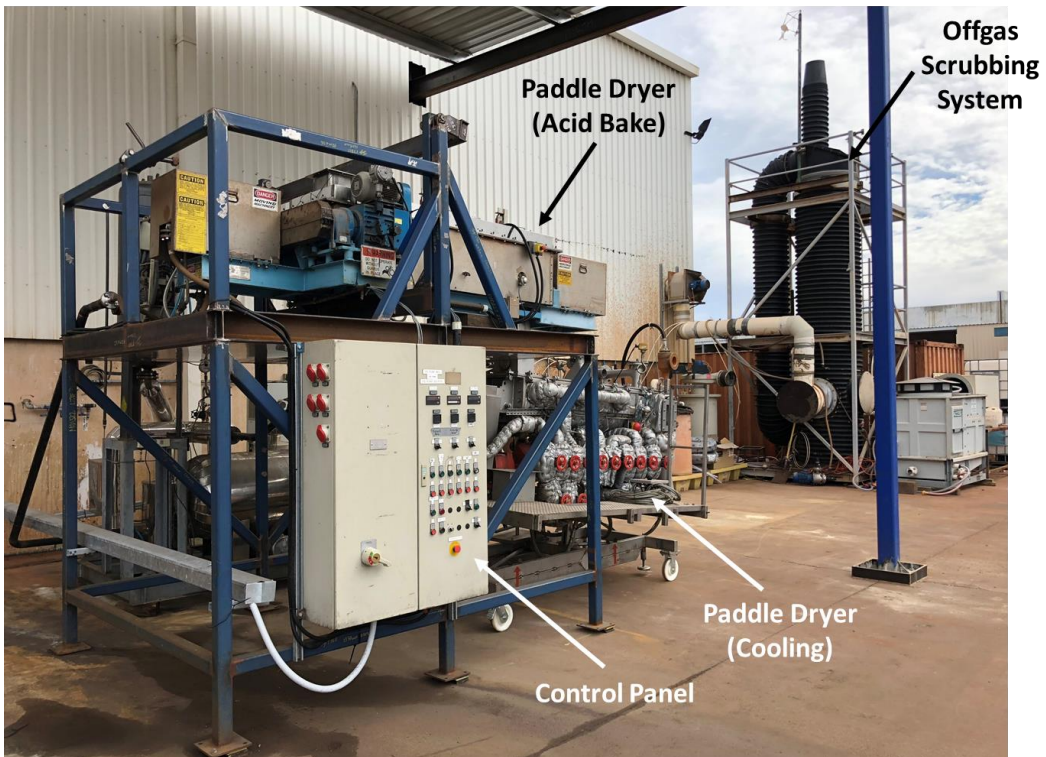
Figure 2b: Phase 4 Acid Bake Pilot Plant at SGS Awaiting Installation of PLR Feeder and Pug Mixer
