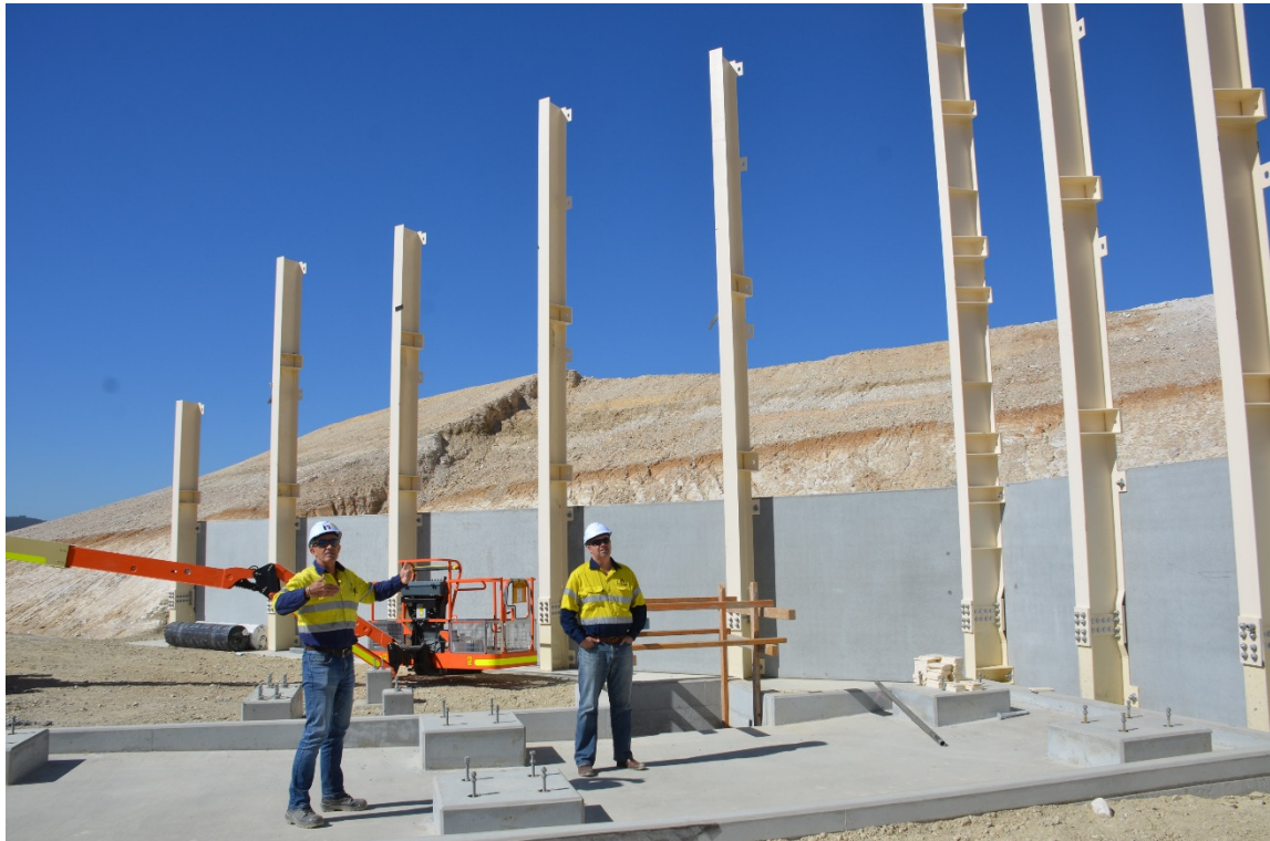
Figure 4: Primary crusher foundations, ROM retaining wall with first lift of panels in place.
