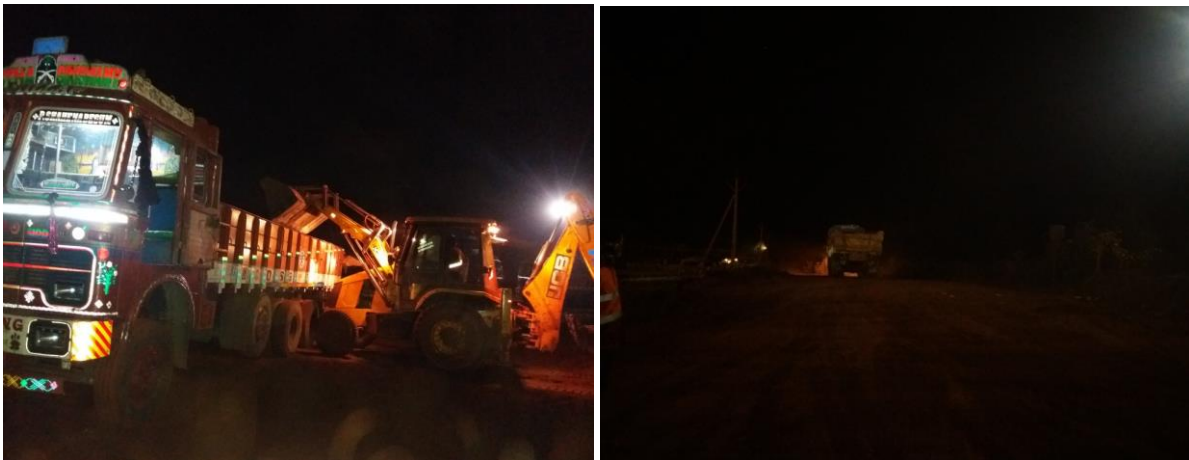
BMM Truck loading and dispatch
