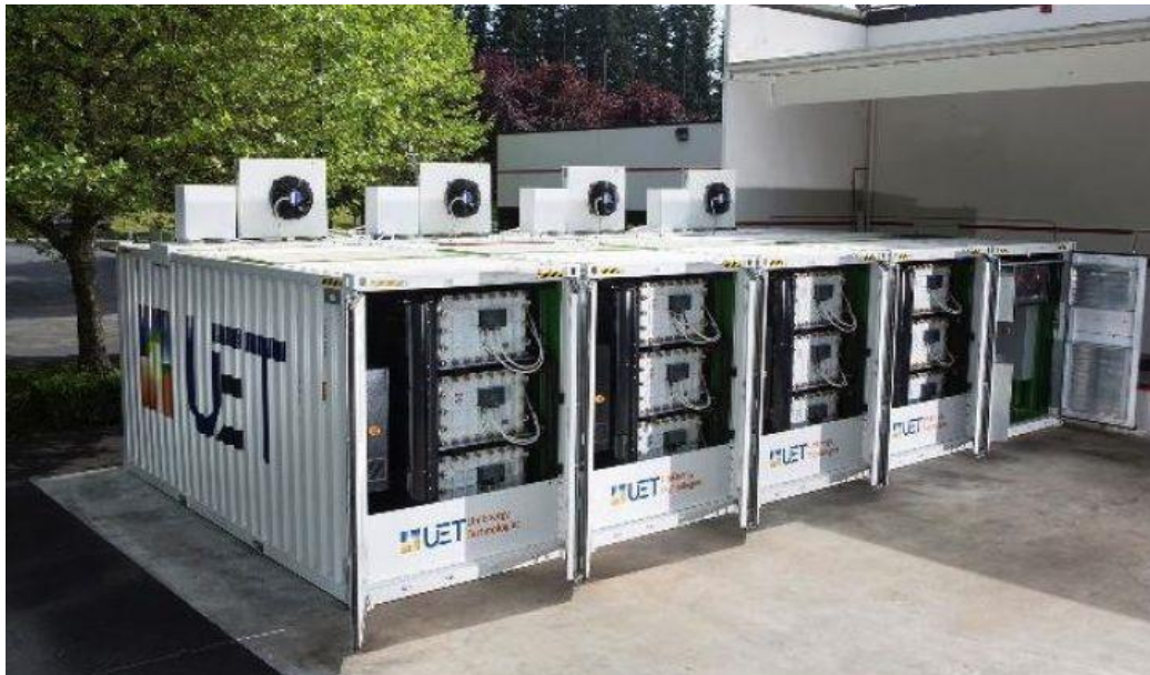
Vanadium redox flow battery storage
