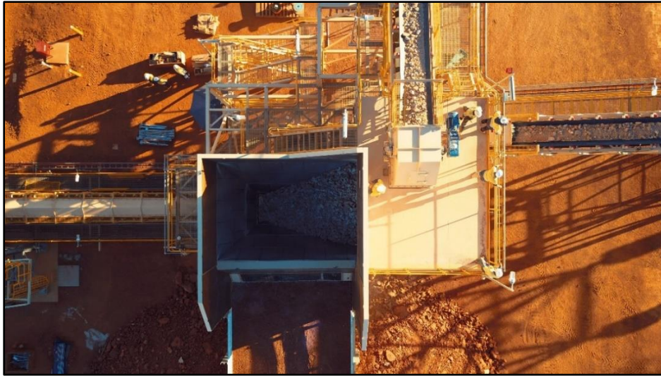
Photo 4: Ore Transfer Bin Commissioned and Fully Operational
