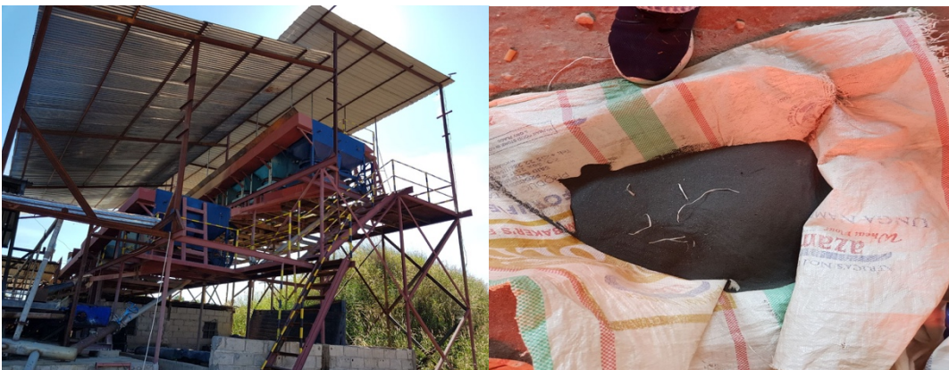
Jig recovery plant and concentrate produced from the plant (PE 13081)
