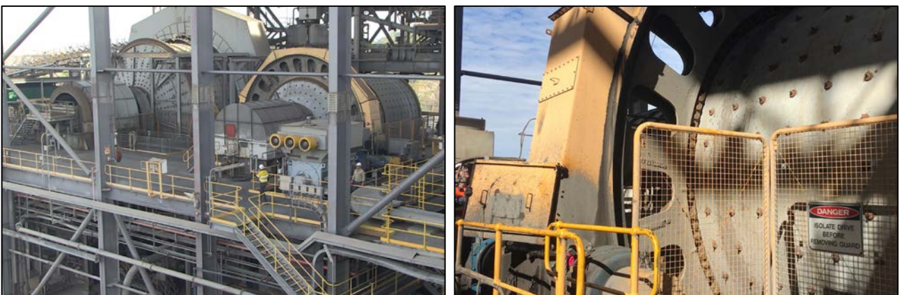
Figures 13 & 14: Ball Mill inspection, refurbishment and inching run completed in preparation for commissioning in July on receipt of first fills of grinding media
