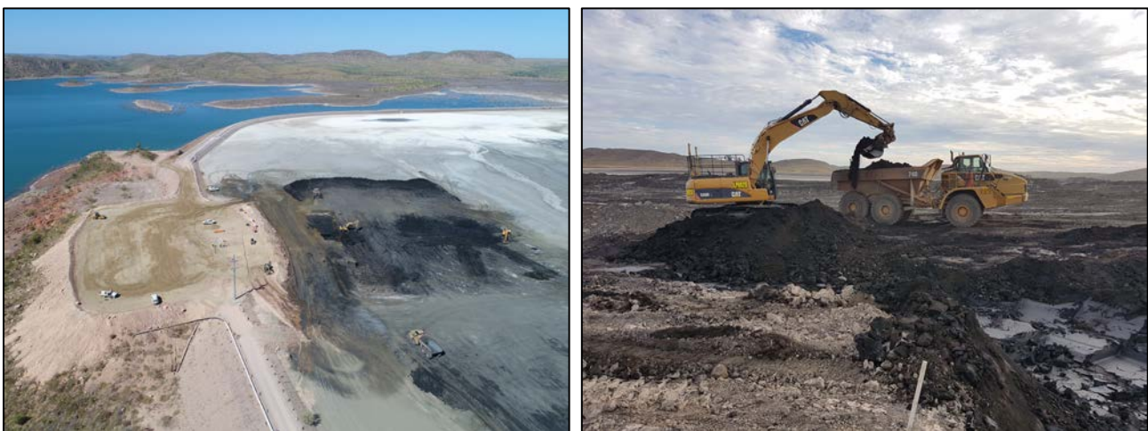
Figures 3 & 4: Aerial view of the hydraulic mining area with evaporation dam in the background (left) and Tailings Slurry Receival Sump excavation activities (right)
