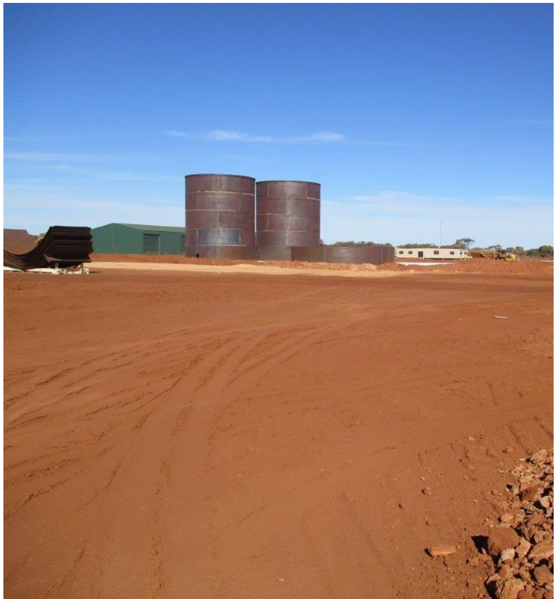
Cardinia Site - 28 May 2018. Partially complete leach tanks with warehouse and offices in the background.
