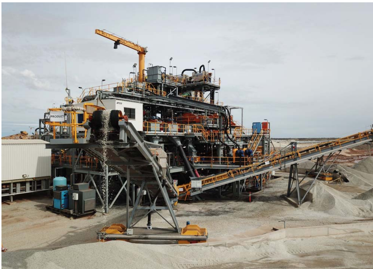
Figure 3: Stage 1 DMS Plant
