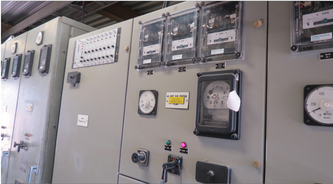
Figure 5 – MCC in Project Substation (Superior 2018)
