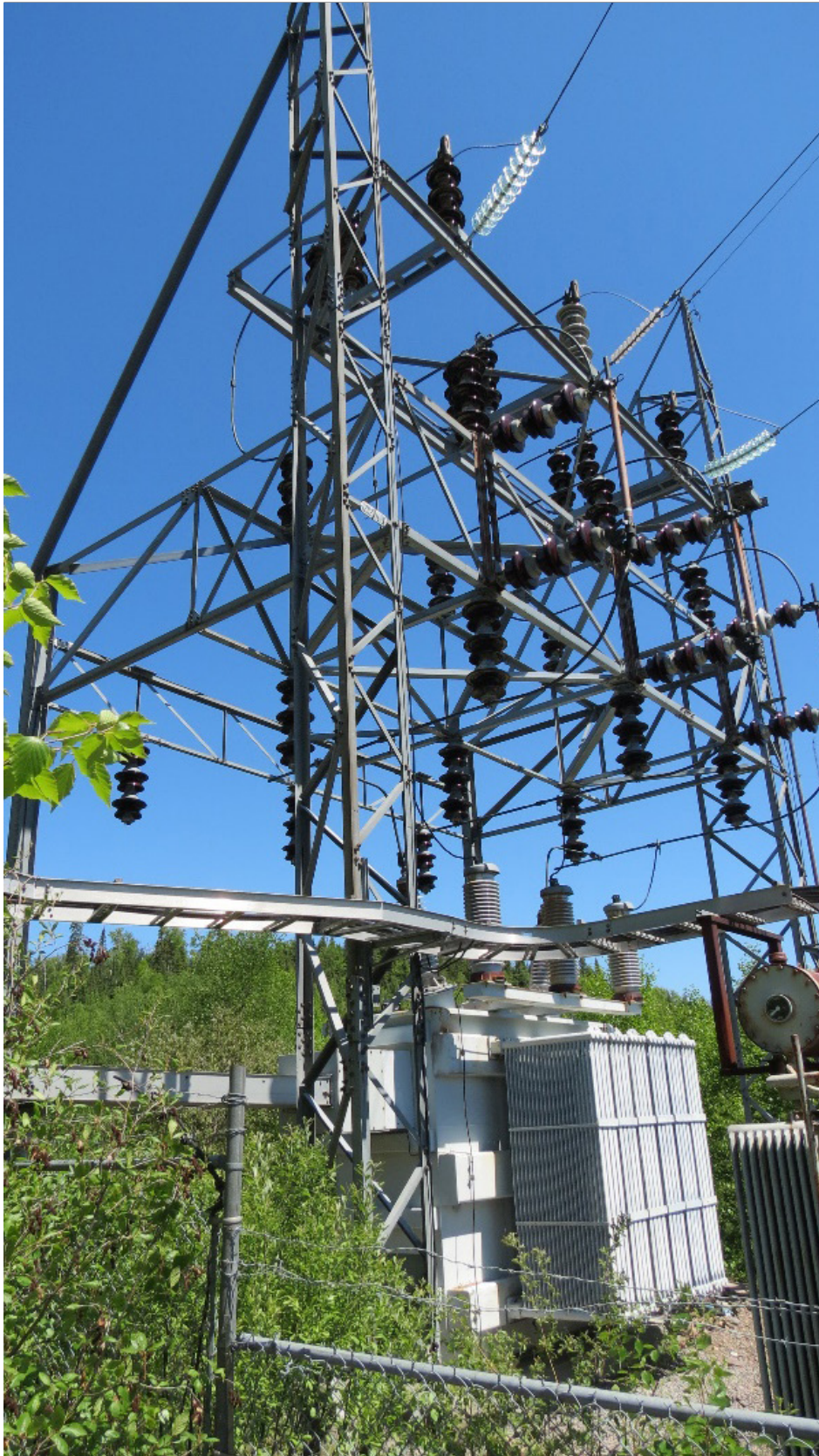
Figure 4 – 115kV: 44kV Transformer (Superior 2018)
