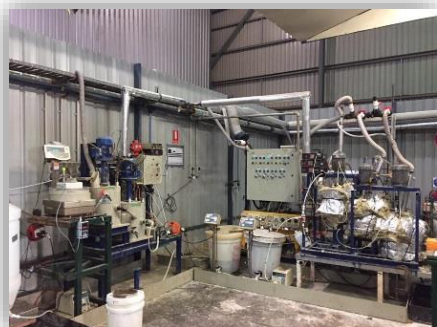
Phosphate Extraction Pilot Plant
