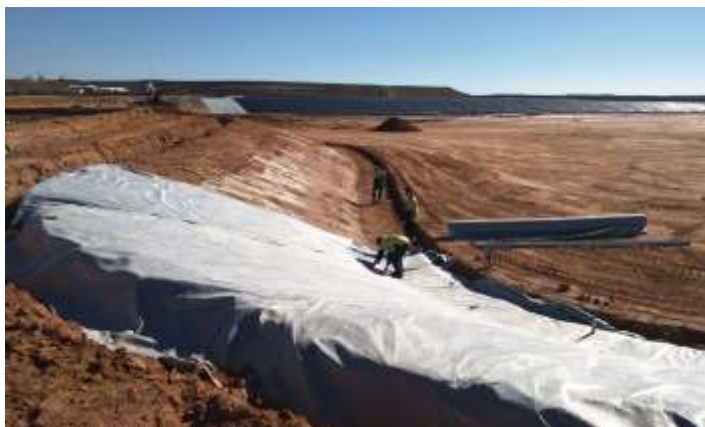
Lining WMP 2 – installing the geotextile underlay in preparation for the HDPE liner
