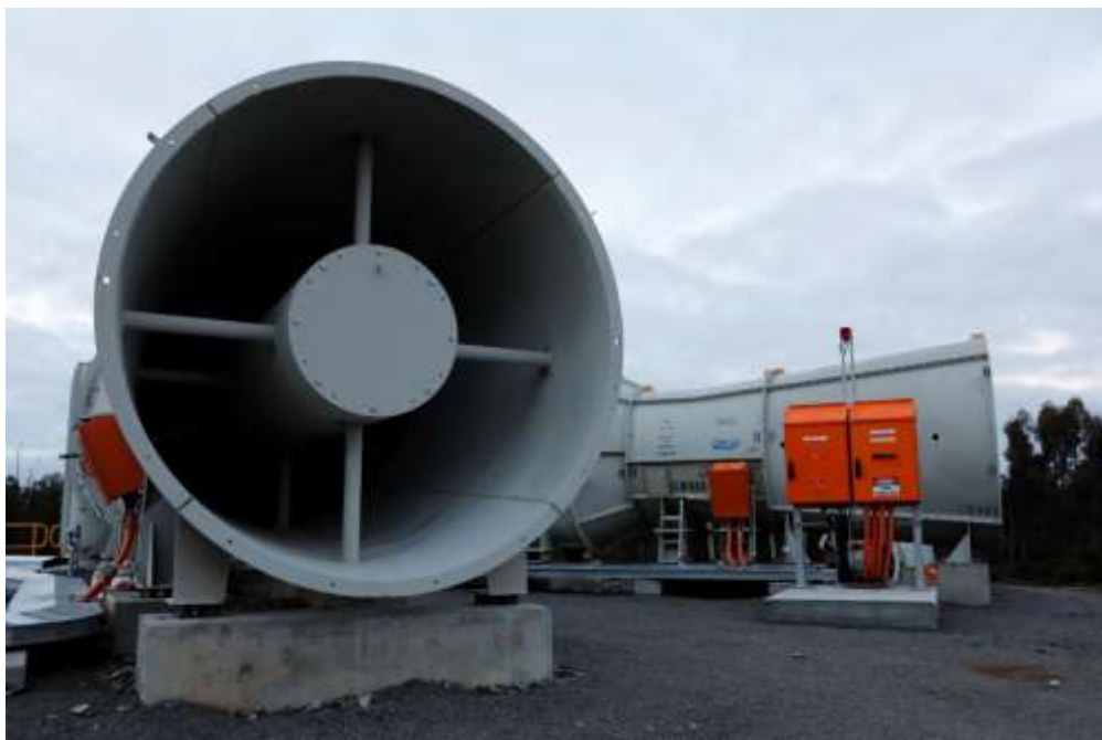
Primary surface fans installed at Spotted Quoll
