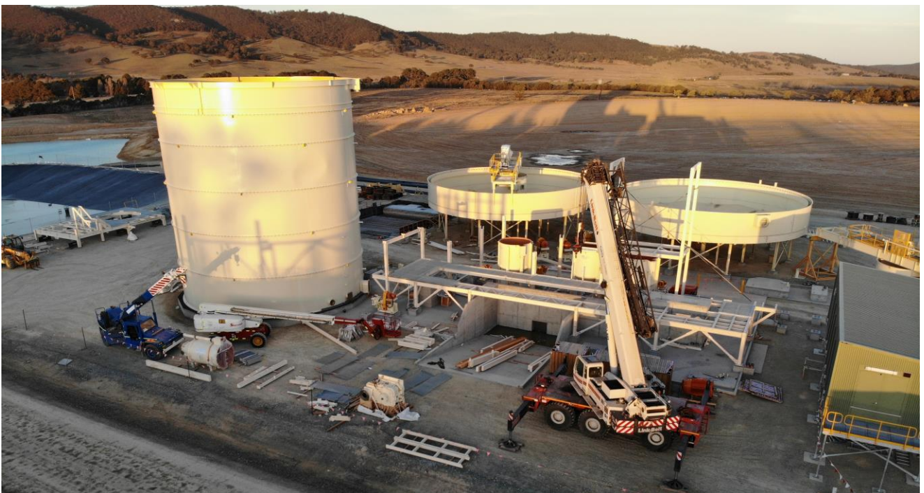
Figure 3: IsaMill™ feed tank and foundations. Tailings and reclaimed tailings thickeners (background).
