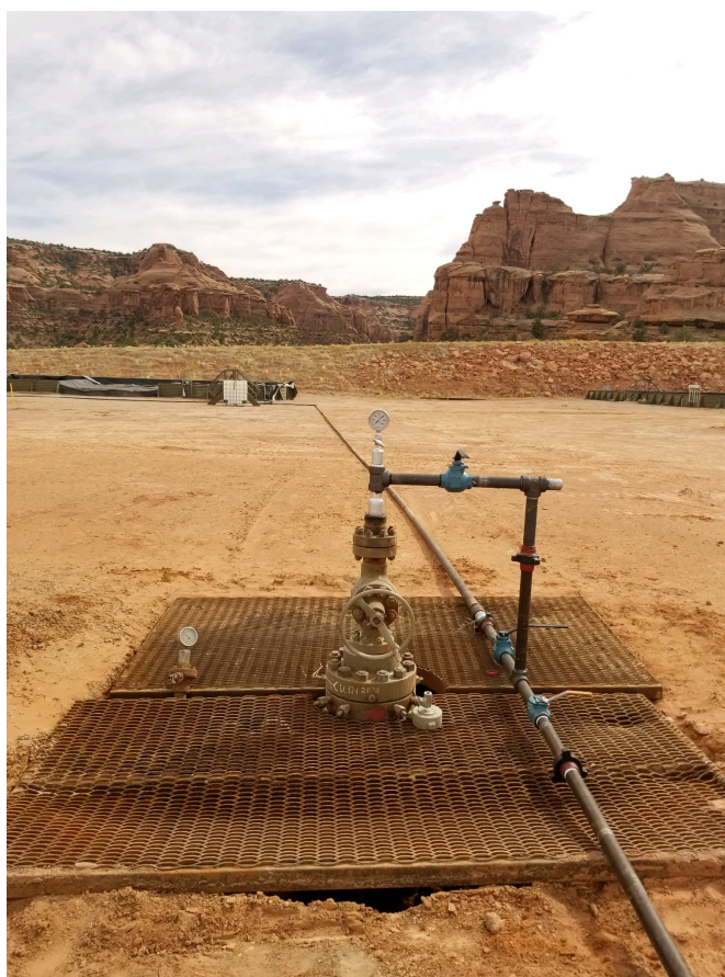
Figure 4: The Cane Creek 32-1 well head.
