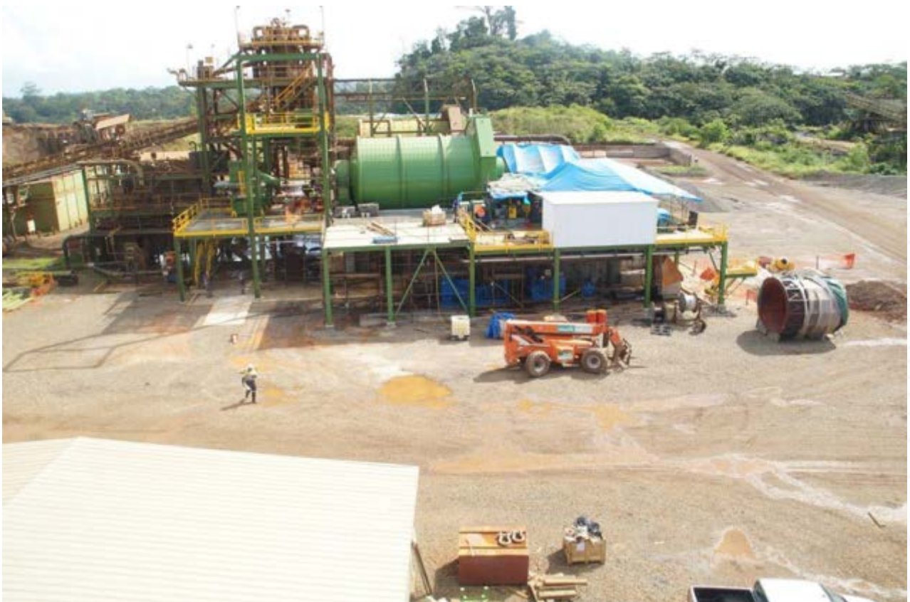
Figure 3. View to grinding section of plant showing ball mill in foreground and SAG in background
