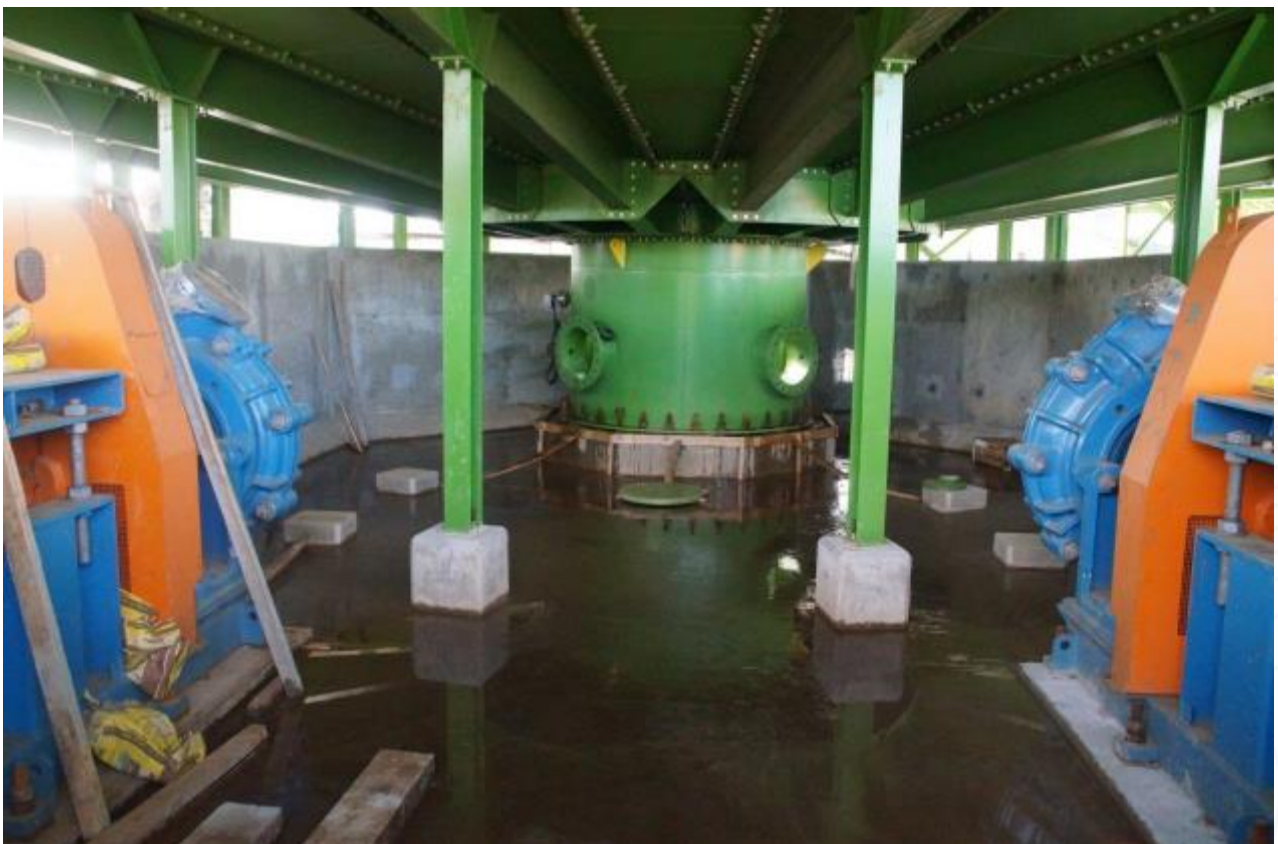
Figure 5. Pre-leach Thickener under flow and pumps
