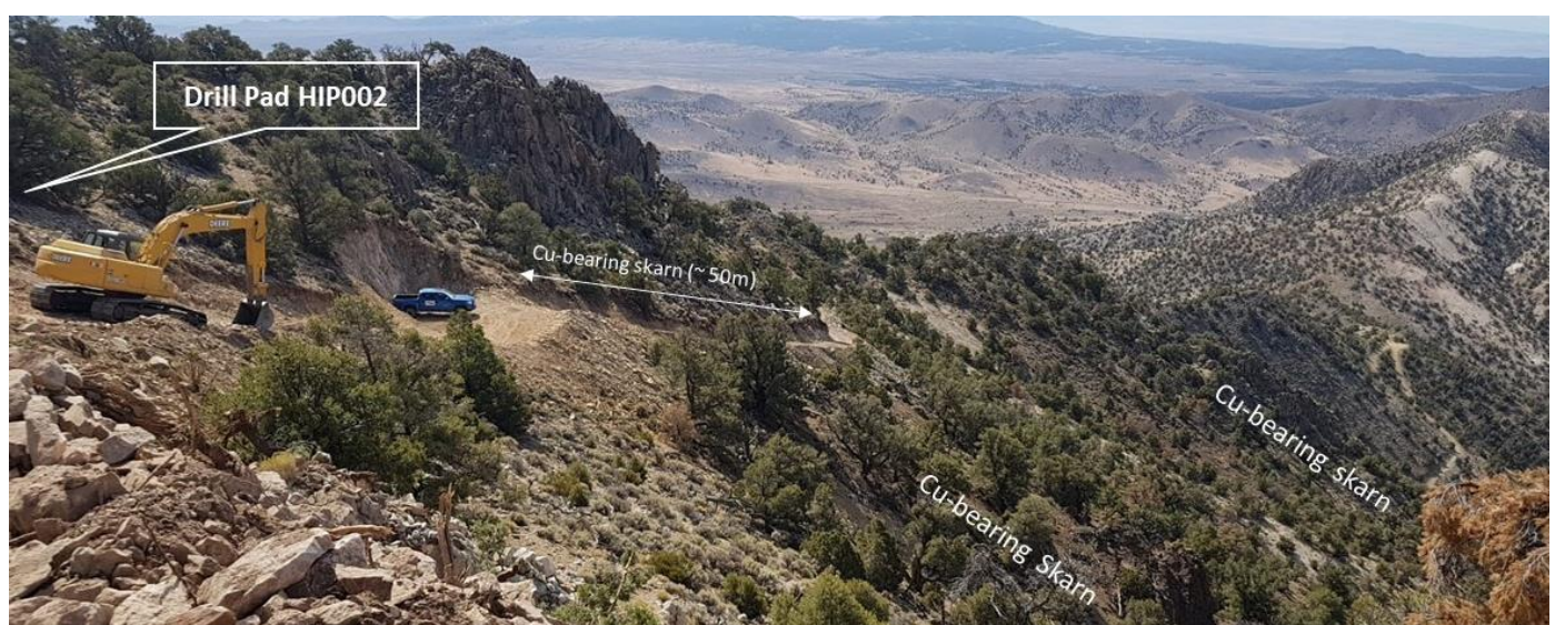
Figure 2: Roadworks and drill pads nearing completion. At least seven drill holes for up to 3000m are planned from drill pads HIP002-HIP004 along the Upper Accrington road as part of an overall 7000m program.
