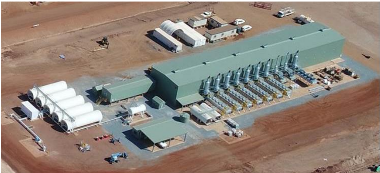
Figure 11: Pilgangoora power station
