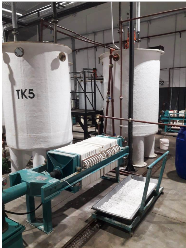
Figure 2. Rincon Lithium Project – Stage 1 Industrial Scale Pilot Plant with initial ‘Battery Quality’ LCE product
