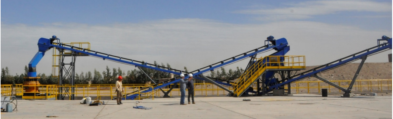
Figure 2 | Vista Gold Plant primary crushing circuit, adjacent to stockpile receiving, and fine ore stockpile and blending area.
