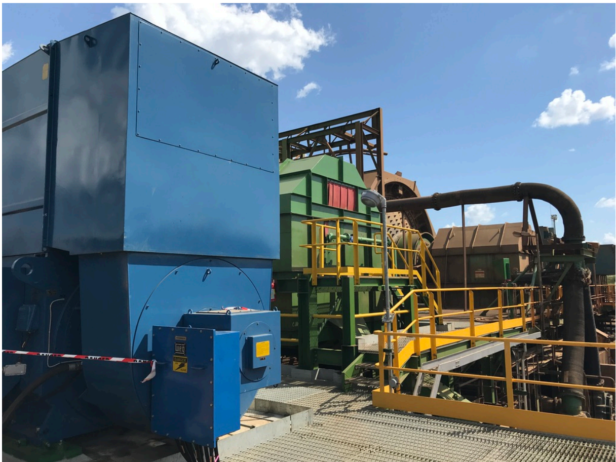
Figure 5. Ball mill motor (foreground) and ball and SAG mill discharge (trommel)
