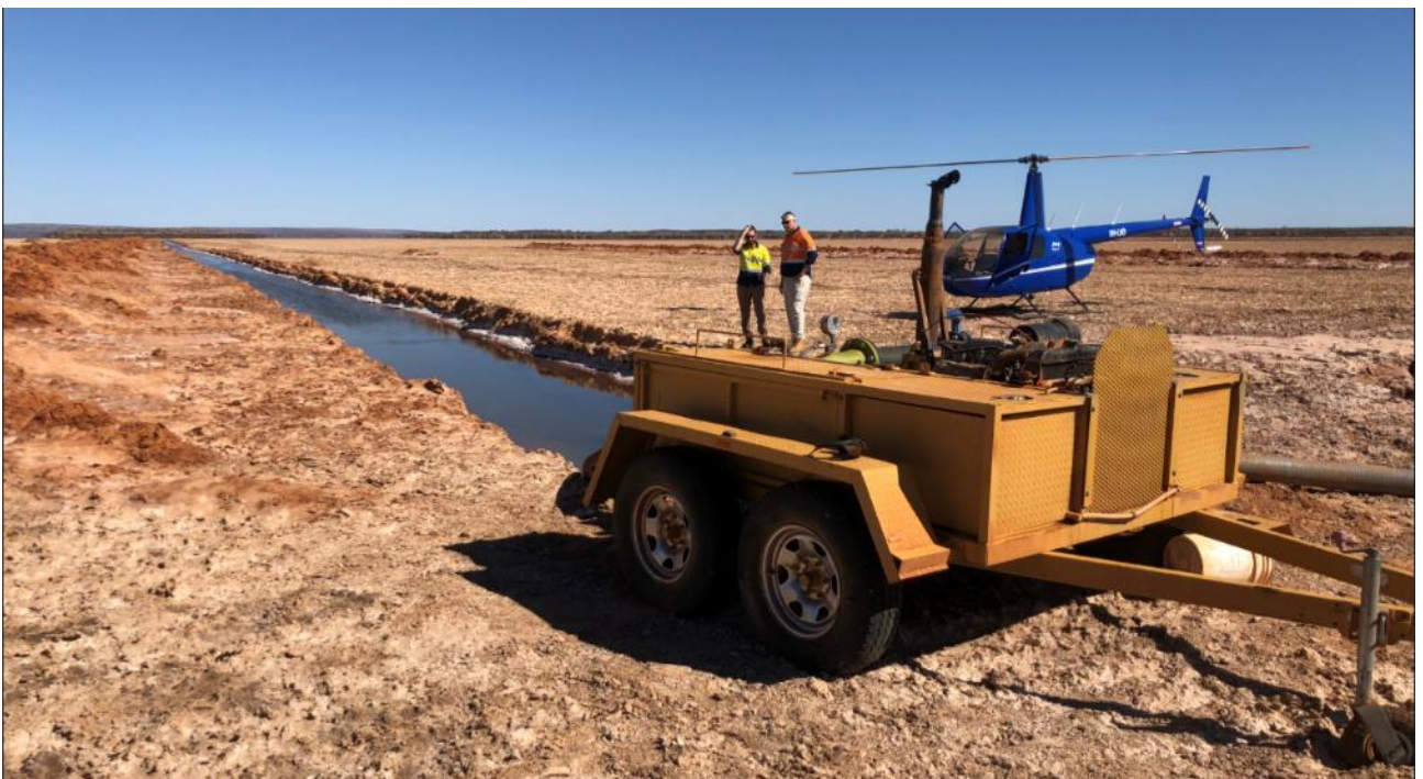
Figure 66: Existing trench pumping set-up [26]
