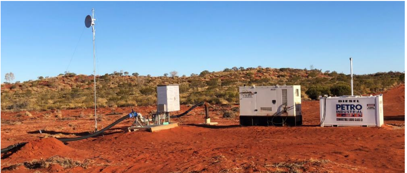
Figure 65: Existing production bore set-up [26]
