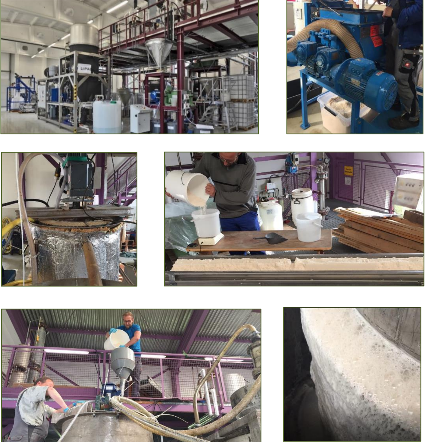
Figure 41: K-UTEC Pilot Plant Facilities [25]
