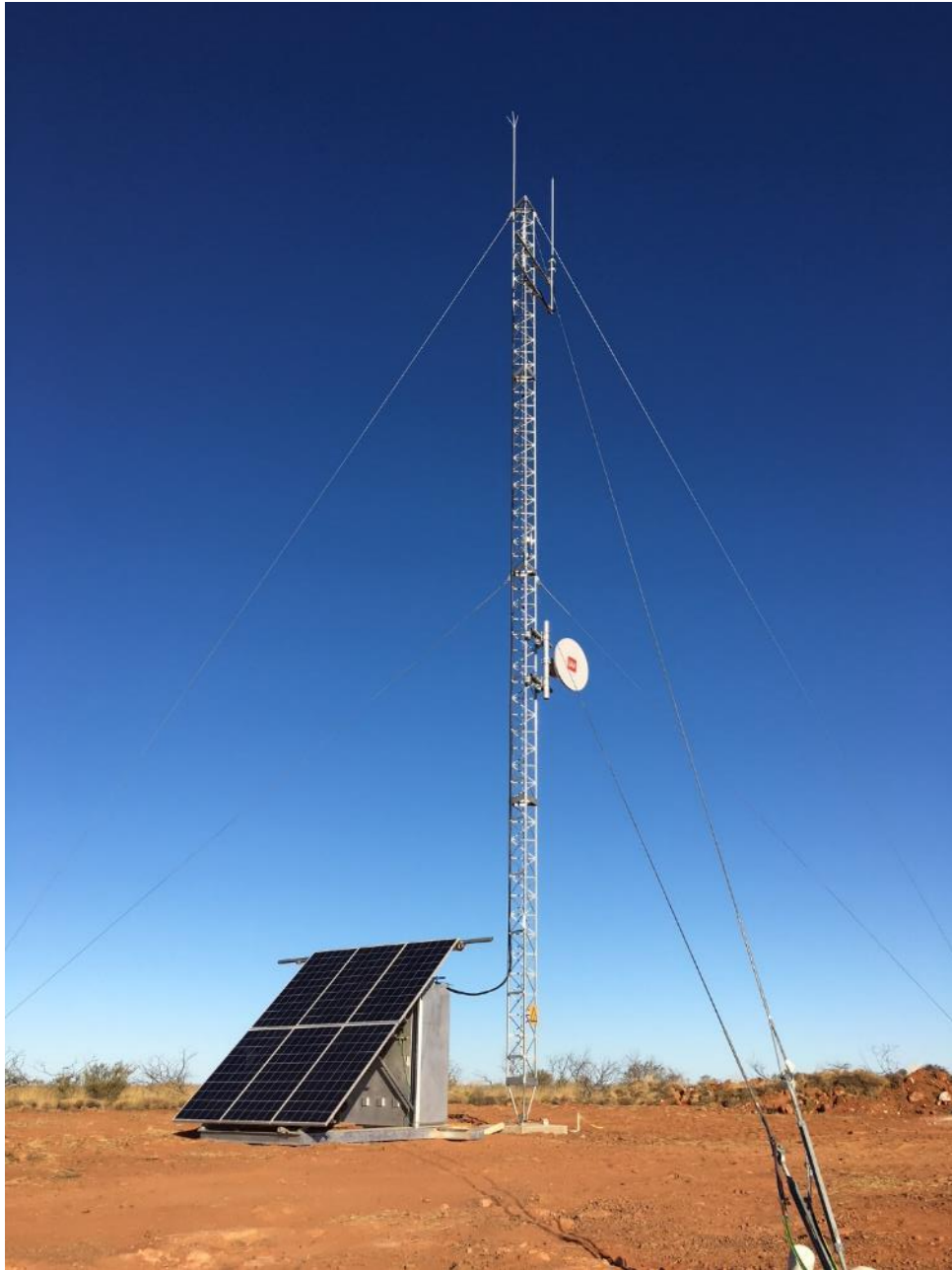
Figure 77: Installed Communications Tower [26]
