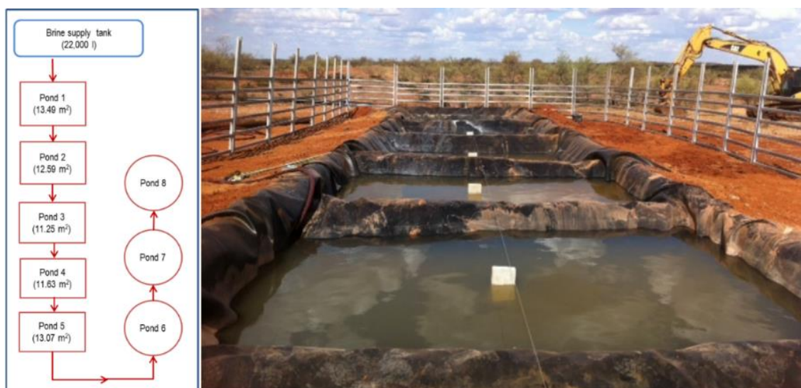
Figure 34: Small Scale Pilot Evaporation Ponds [3]
