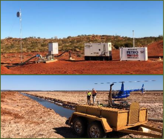
Brine Pumping from Bores and Trenches >260 Million litres successfully pumped to date
