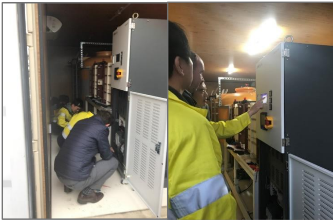
KORID technicians overseeing installation of the V-KOR battery at the Perth test site
