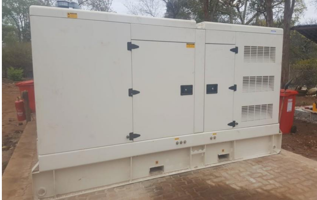
The 2 x 500 KVA generators that will power the new camp have arrived on site
