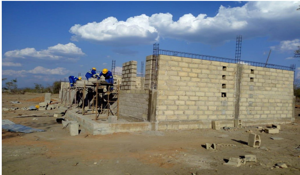
Battery Minerals is building a school for the Ministry of Education, located in the Village of Nkawene which serves over 600 pupils
