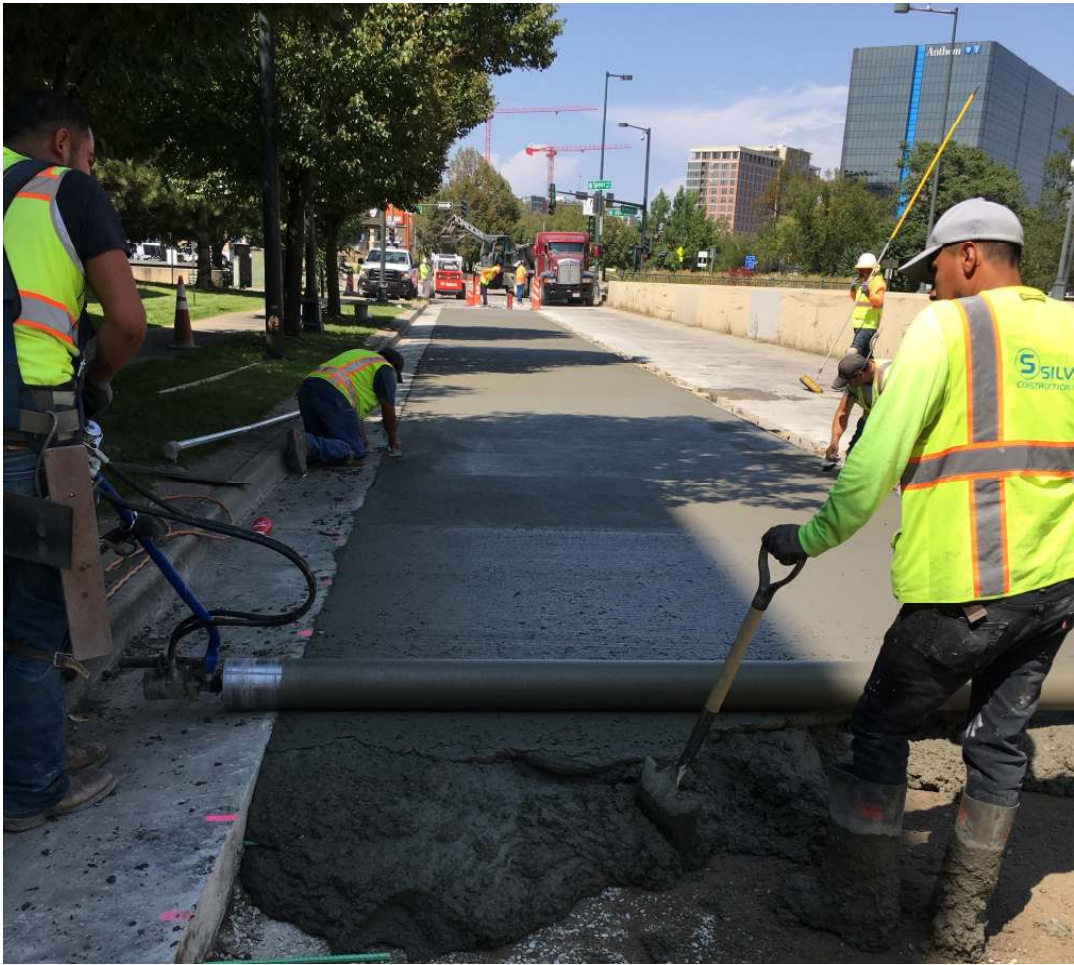
Figure 2 – One of Two New Trial Sections of Concrete Pavement in second trials
