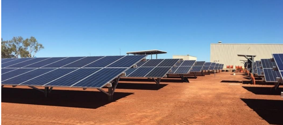
Delamere Microgrid Project
