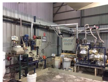
Phosphate Extraction Pilot Plant
