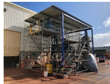
Acid Bake Pilot Plant
